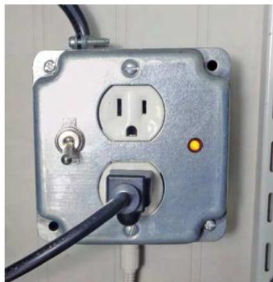
Figure 3 — Astron Corporation power supply remote-control interface with bypass switch.
