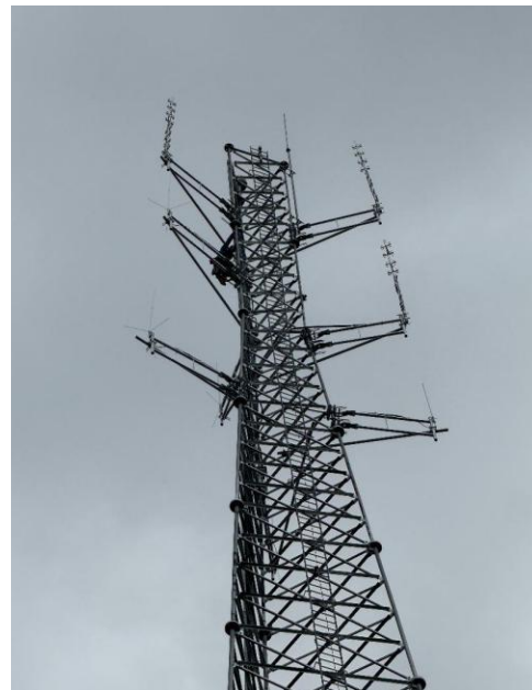
New Tower with Club Antennas
